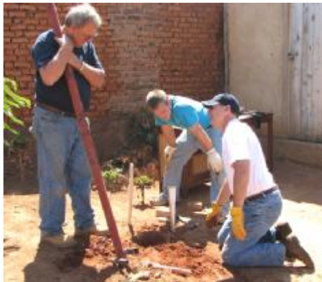
Frank Strickland, left, works with Caleb Owen, center, and Kip Miller as they begin to construct a drying shed at the Children's Home.
